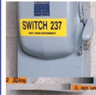
Panel & Switch I.D.
