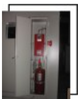
Fire Suppression System
